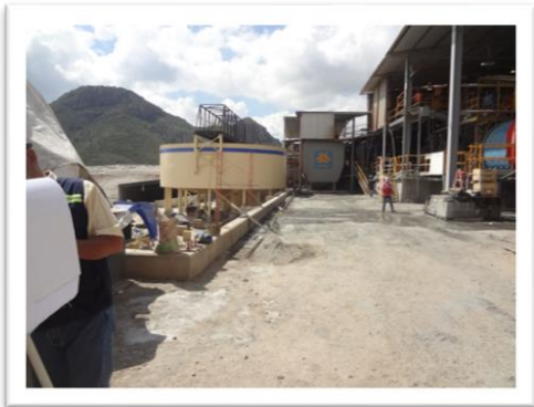
New Thickener tank
