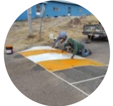
Street and road maintenance and Landfill cleaning was carried out in the communities of Panuco de Coronado, San Jose de Avino, and Zaragoza
